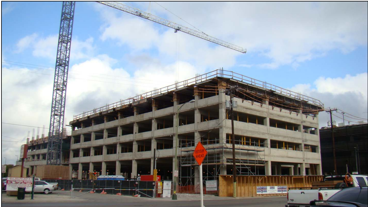
Bexar County is now constructing a Flores Street Parking expansion to accommodate the Justice Center Expansion employees and customers with 500 additional parking spaces. The parking garage will include an office build-out on the first floor. The project is currently budgeted at $14.6 million
